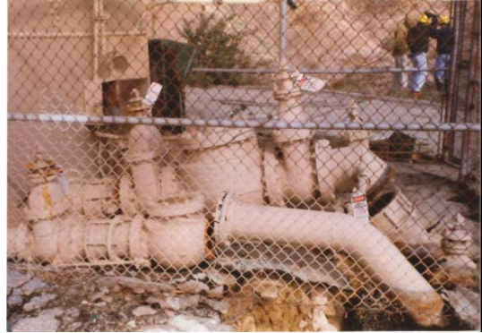
Damaged tank inlet/outlet lines in the 1994 Northridge earthquake. Image courtesy Los Angeles Department of Water and Power.
